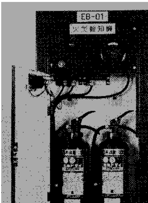
Photo 6.5 A fire extinguisher box with a push button fire alarm in a tunnel in Japan
