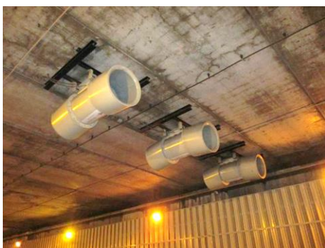
Figure 11 - jet fans in the ceiling
