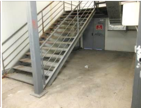
Figure 9 - ascending escape staircase
