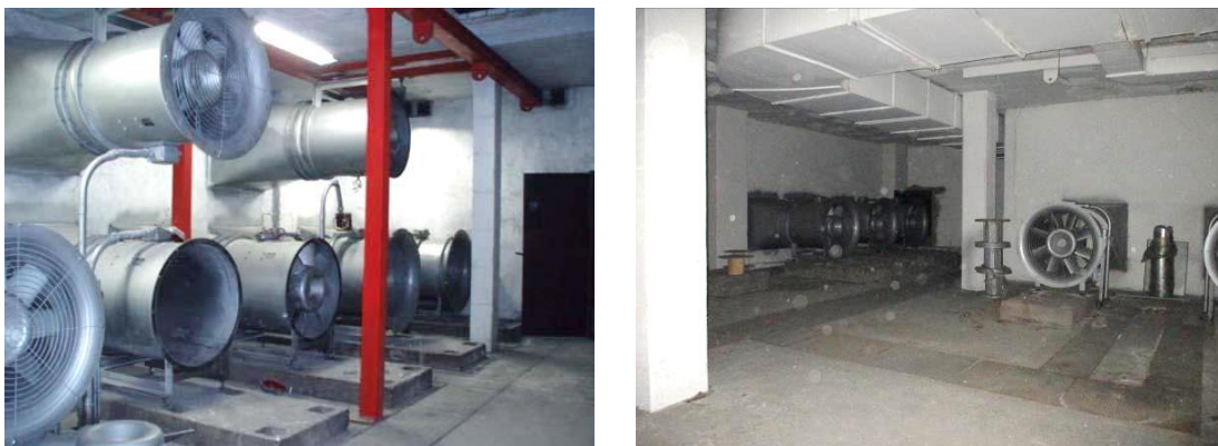
Figure 7 – Tunnel ventilation stations
