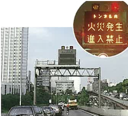
Figure 3 - Warning Sign Board
