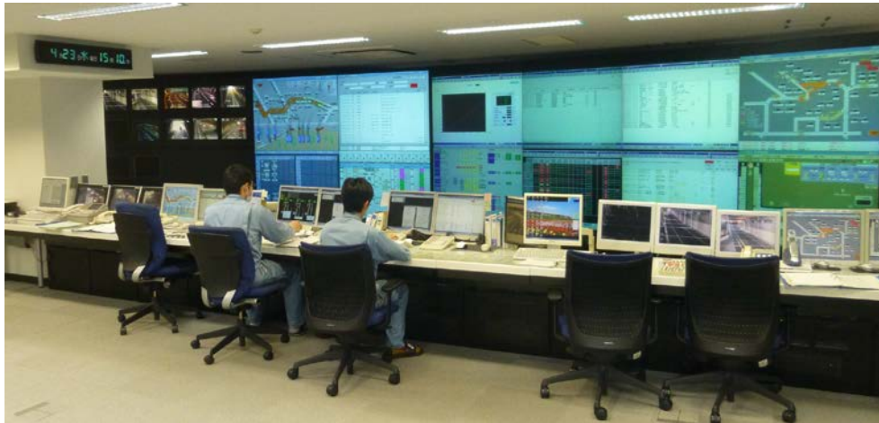
Figure 12 – Operation Room in the Hirakawa-cho Ventilation Station
