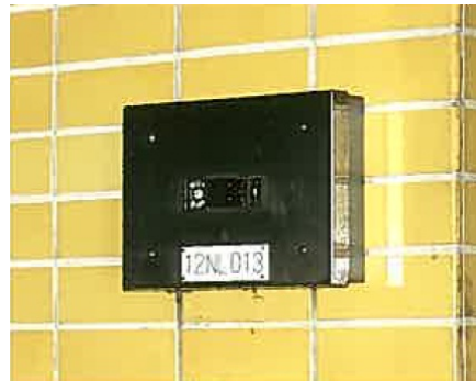
Figure 6 - Automatic Fire Detector
