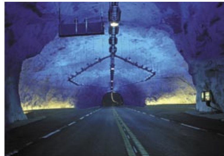
Figure 28: Tunnel interior of a Norwegian tunnel with orientation lighting
